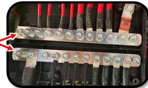
Main Fuse Testing Points
